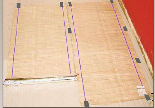
2. The foil strip heater is unrolled on top of the foam underlay and secured with tape.
